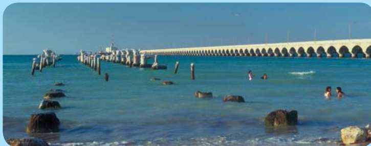
Concrete piers with mild steel re-bars after 32 years of service (left) and stainless steel re-bars after 60 years (right) (Courtesy of Nickel Institute).
