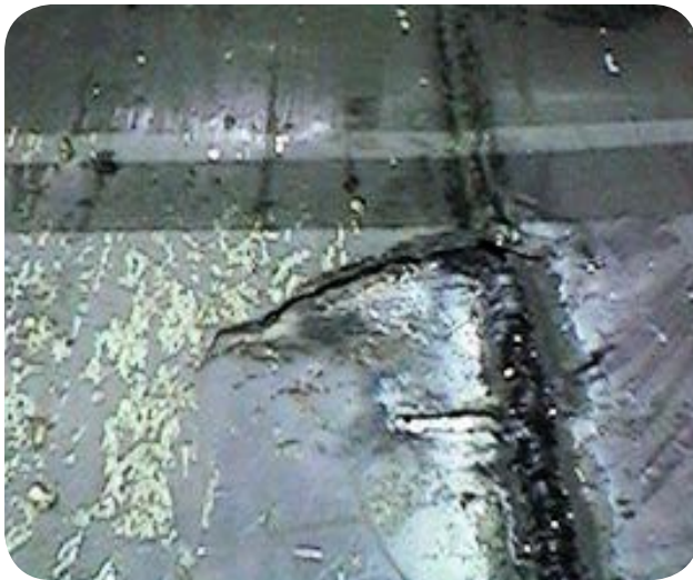
Fig. 2 Thermal fatigue in stainless steel lining.
