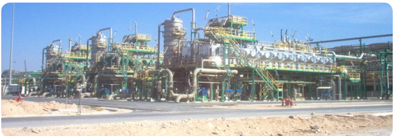
Fig. 7 The first MSF recycling plant with 100% solid 2205 evaporator vessels.
