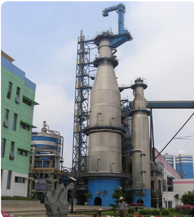
Fig. 4 A continuous kraft digester made of 2205 during erection in China (Courtesy Kvaerner Pulping).
